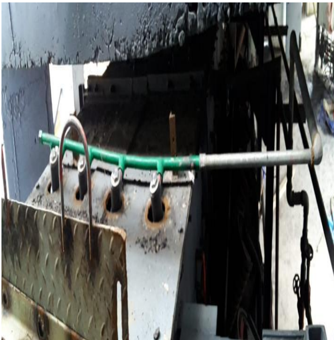
DSS sprinklers at PC-01 Tail end
