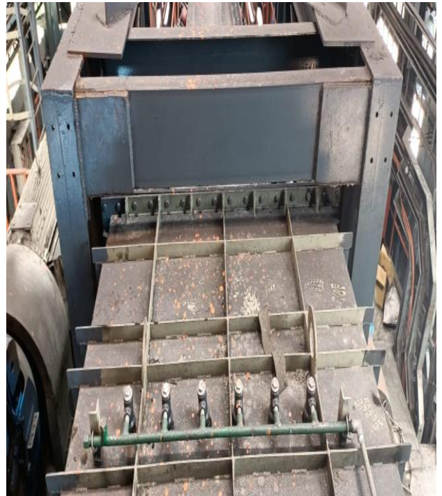
DSS sprinklers at PC Head end
