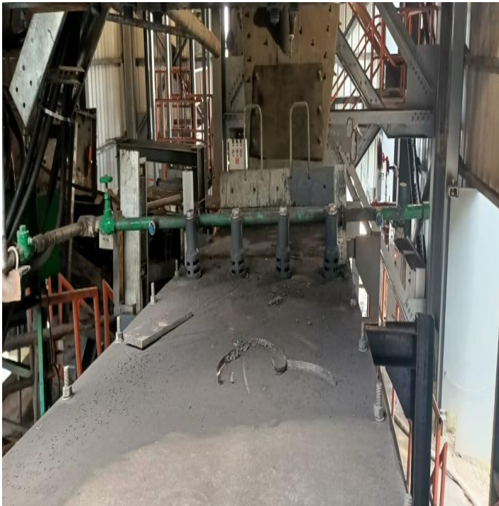
DSS sprinklers at BC-02 Tail end
