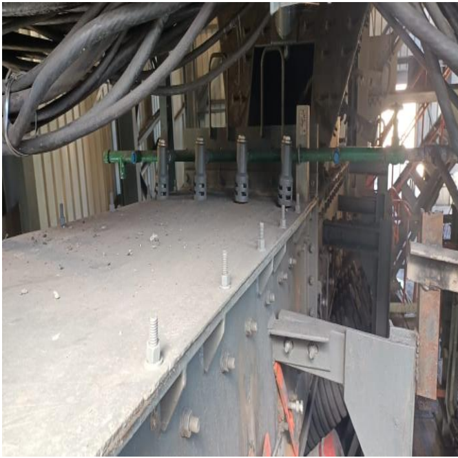
DSS sprinklers at BC-04 Tail end
