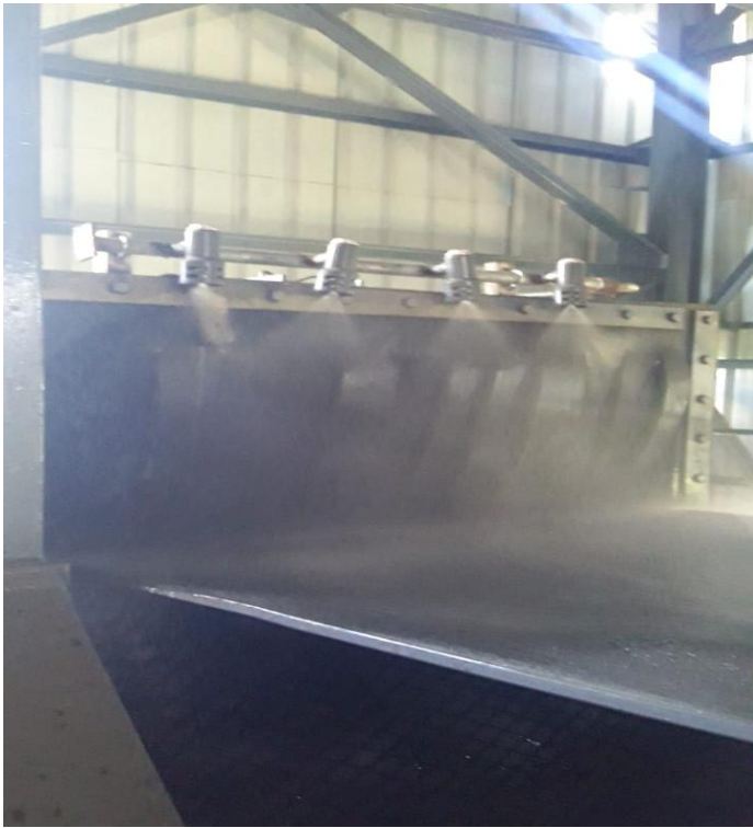
DSS sprinklers at BC-01 Head end
